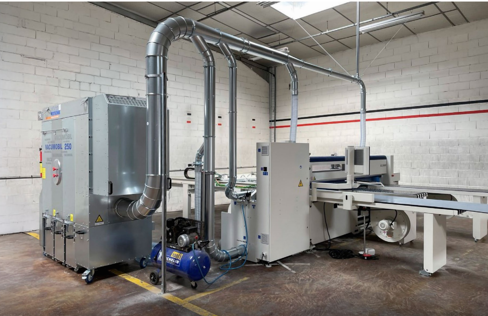
Extraction from a panel saw in plastics processing using the Vacumobil JT 250, discharging into chip bins.
