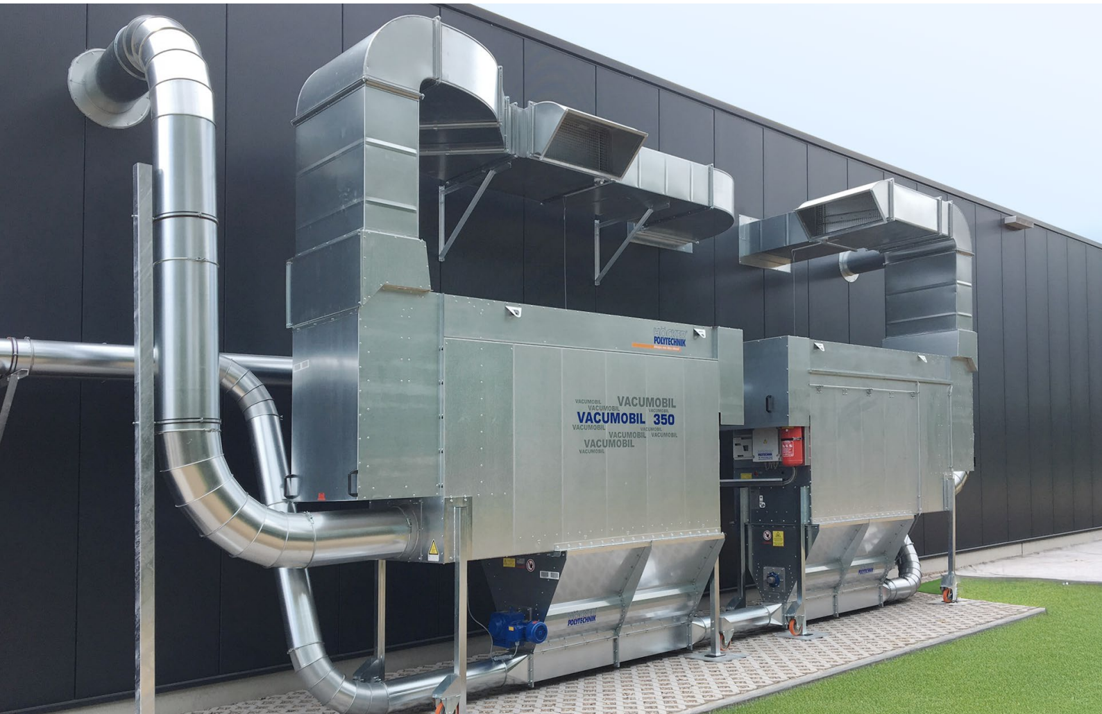
Two Vacumobil JZ 350 units installed outdoors. The cleaned air is returned to production, preserving valuable heat energy.
